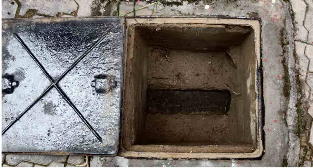
Pic- Groundwater recharge system
