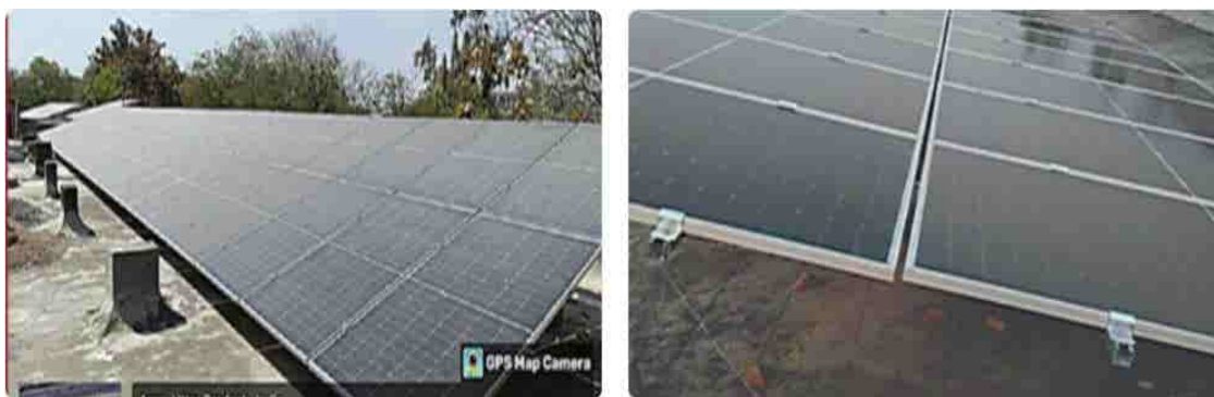
Figure 22: Rows of solar modules on a University rooftop
