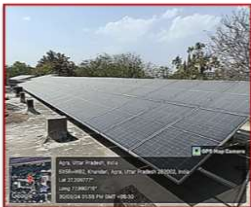
Solar Power System
