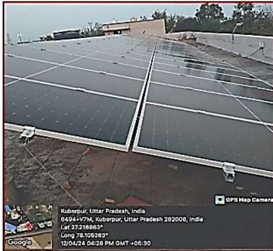
Solar Power System University Campus – 70KWh
