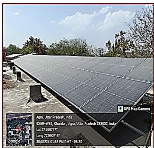
Solar Power System University Campus – 60KWh
