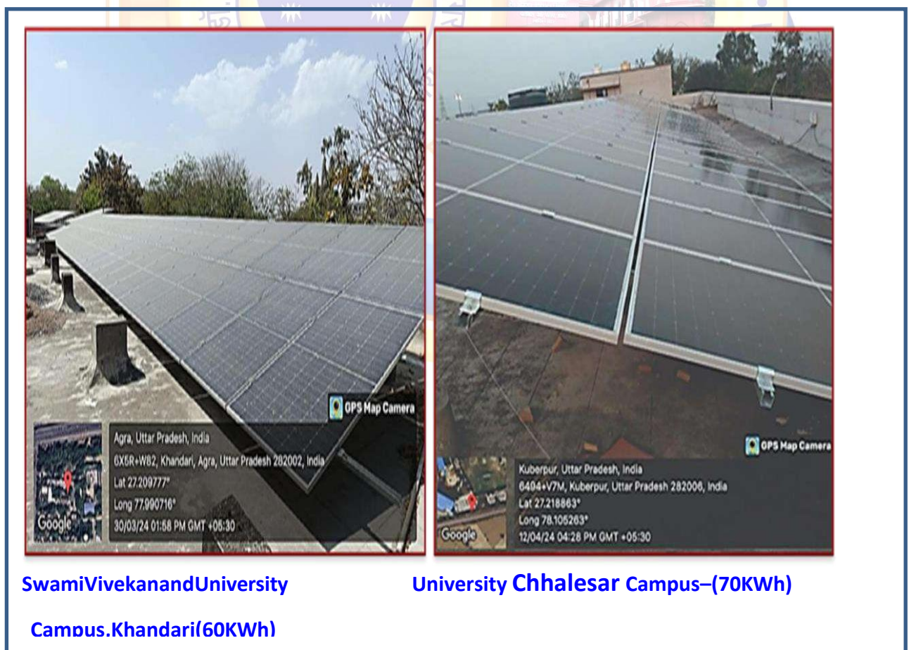
Rooftop solar panels installed at Khandari Campus, DBRAU
